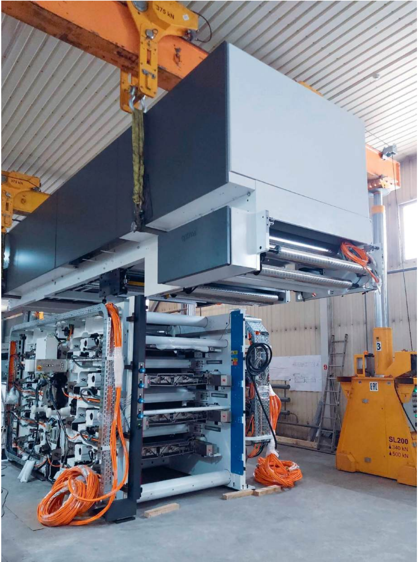
Flexible packaging and polymer products manufacturing in Ust-Kamenogorsk city, East Kazakhstan region. Turnkey installation of a Soma Optima 2 printing press in a low-ceilinged space. GP125 hydraulic gantries.
