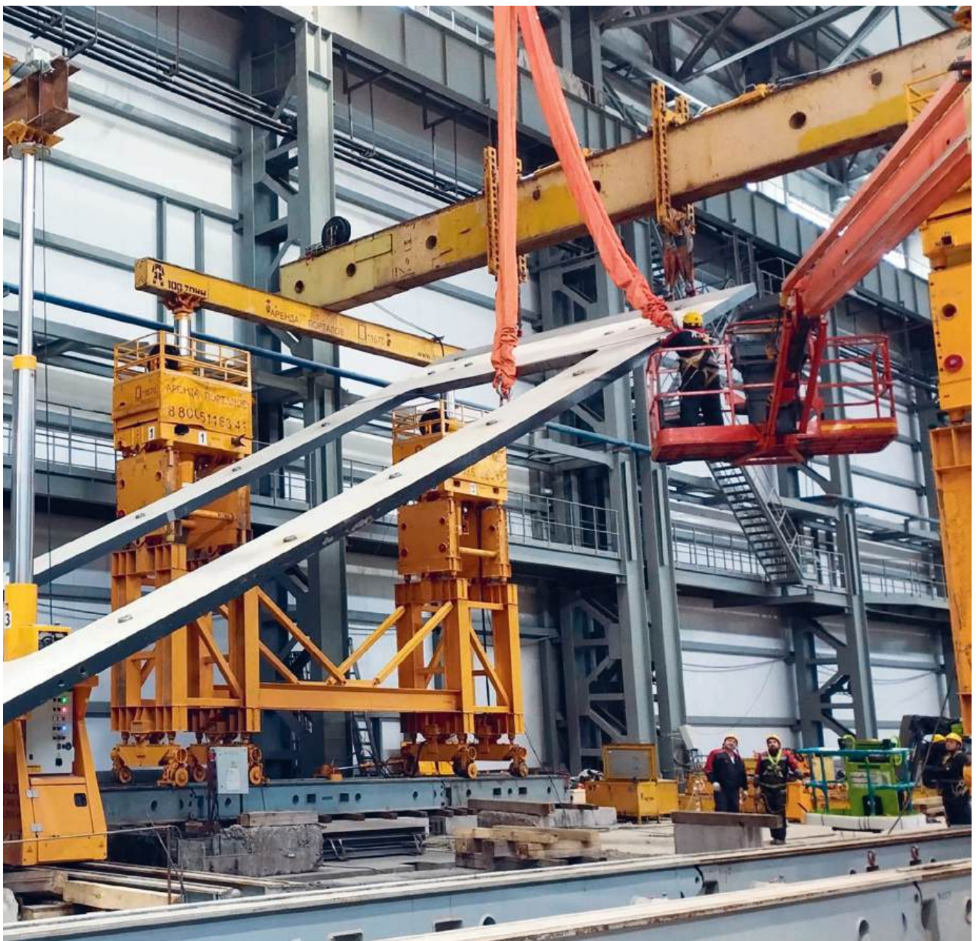
Railway wheel manufacturing plant, Ekibastuz city, Pavlodar region. Assembly of two 890-ton presses and installation of an oil tank. GP500 and GP200 hydraulic gantries.
