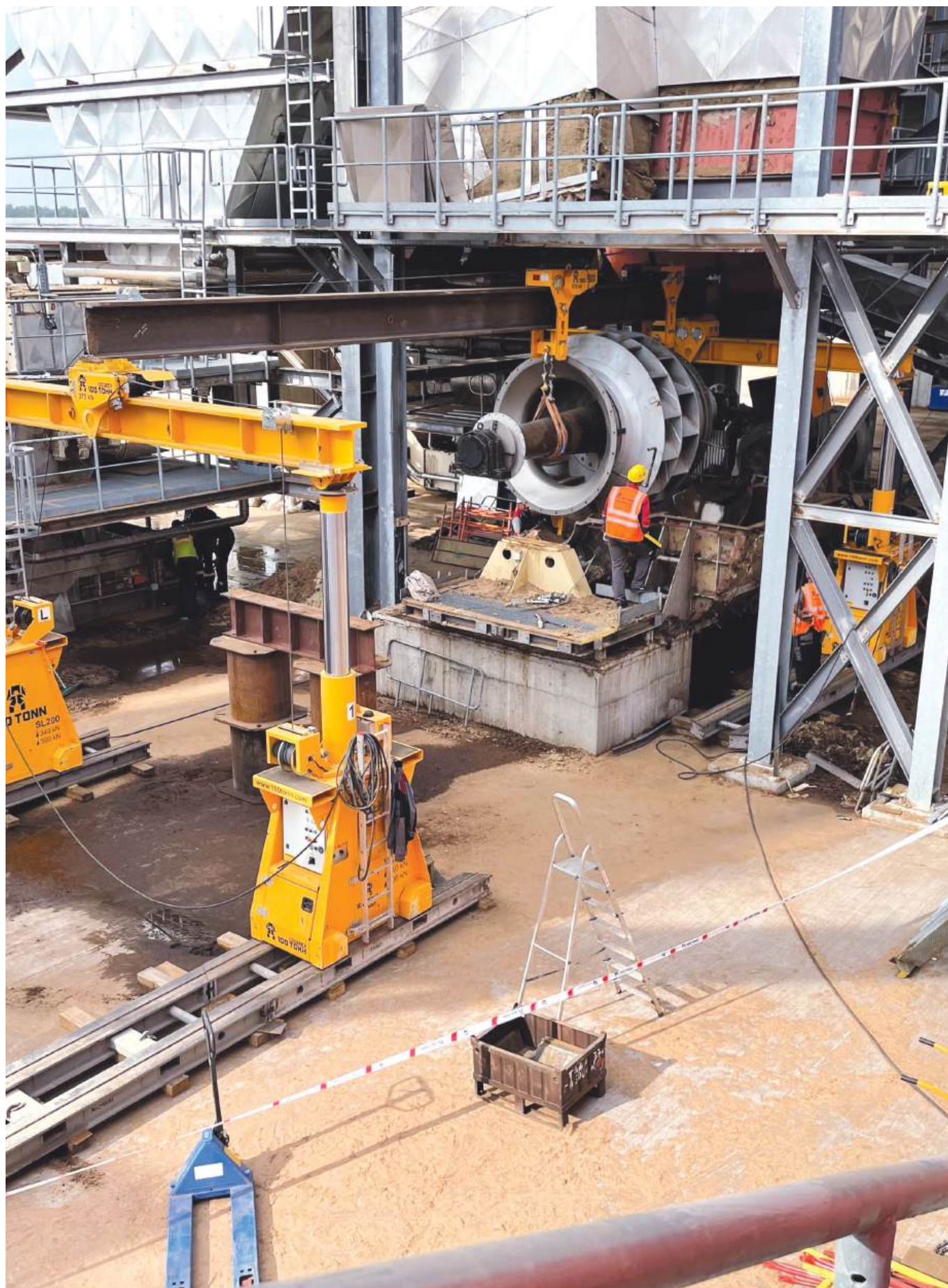
Kronspan plant, Ufa city, Republic of Bashkortostan. Fan impeller removal and installation. GP200 hydraulic gantries.
