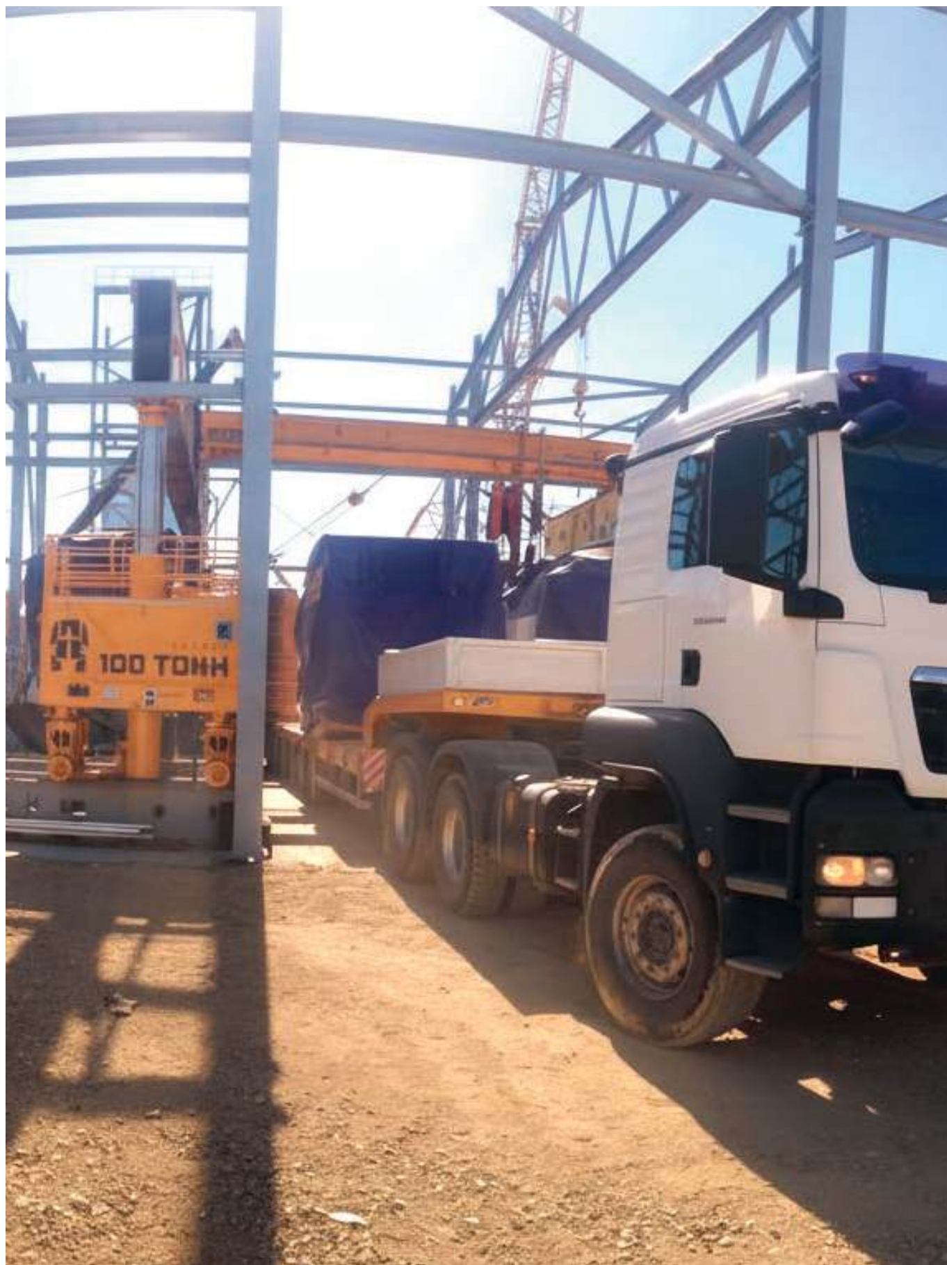
Chemical plant construction in Aktau city. Unloading, decommissioning, pre-assembly, and installation of four Wartsila gas generator units on vibratory supports. GP500 hydraulic gantries.
