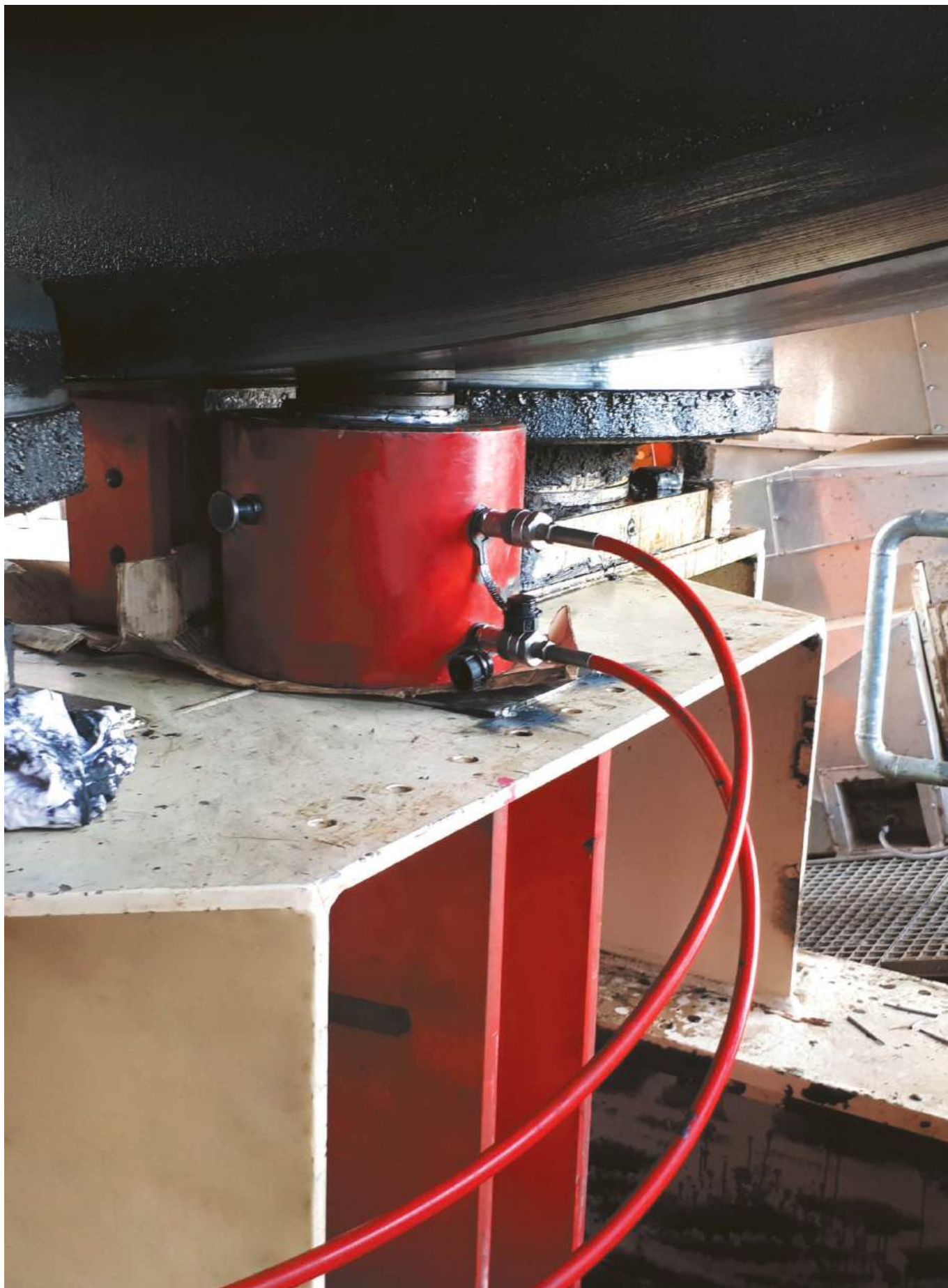
Kronospan plant, Ufa city, Republic of Bashkortostan. Lifting a 450-ton drying drum for repairs.
