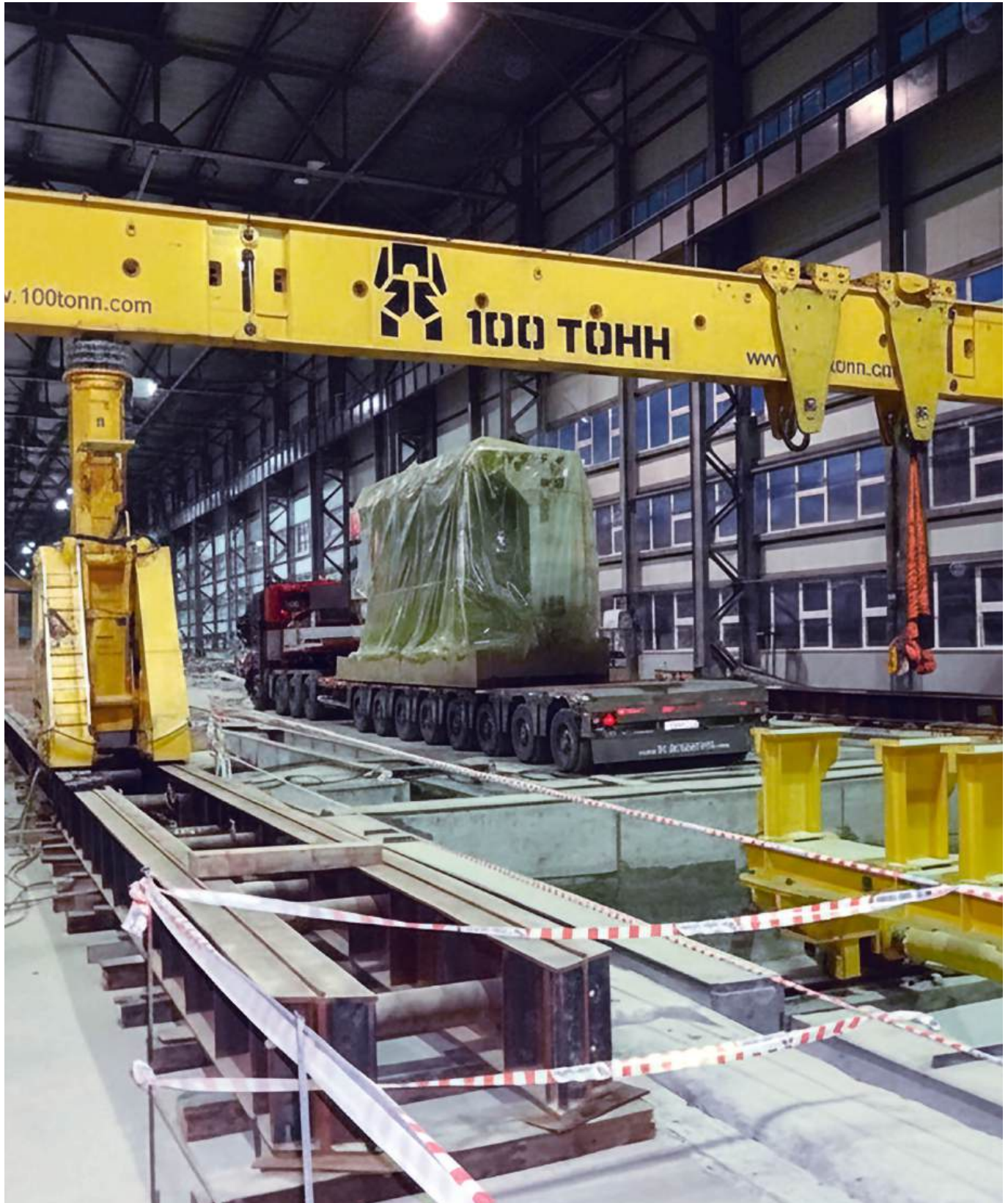
Aktobe Rail and Beam Plant, Aktobe city. Transportation and installation on the basement of horizontal and vertical straightening machines weighing over 100 tons. GP1100 hydraulic gantries.
