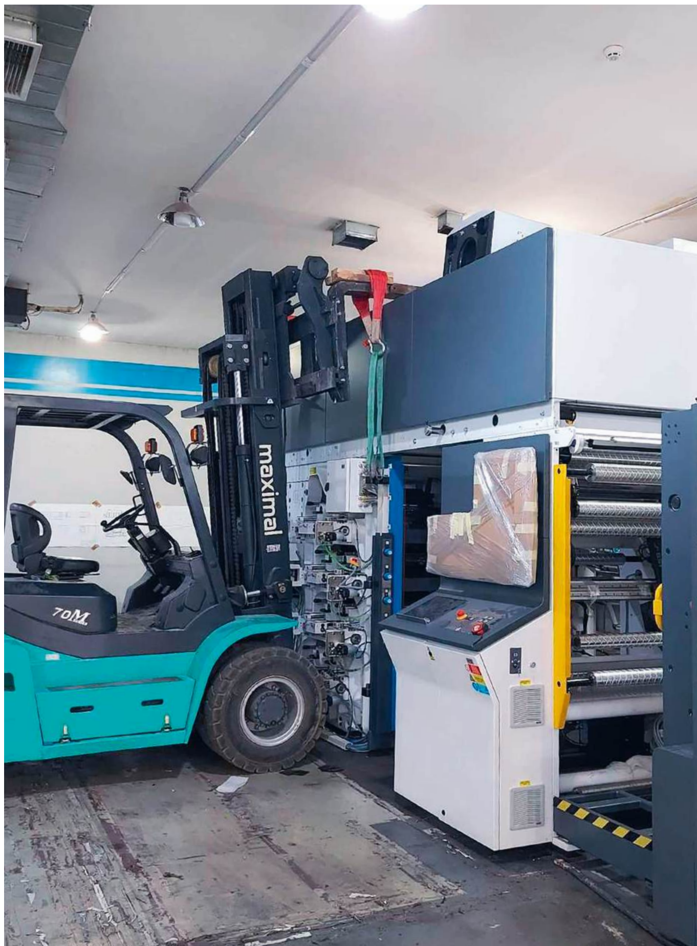
POWERFLEX Printing House, Tashkent city. Turnkey installation of printing equipment.
