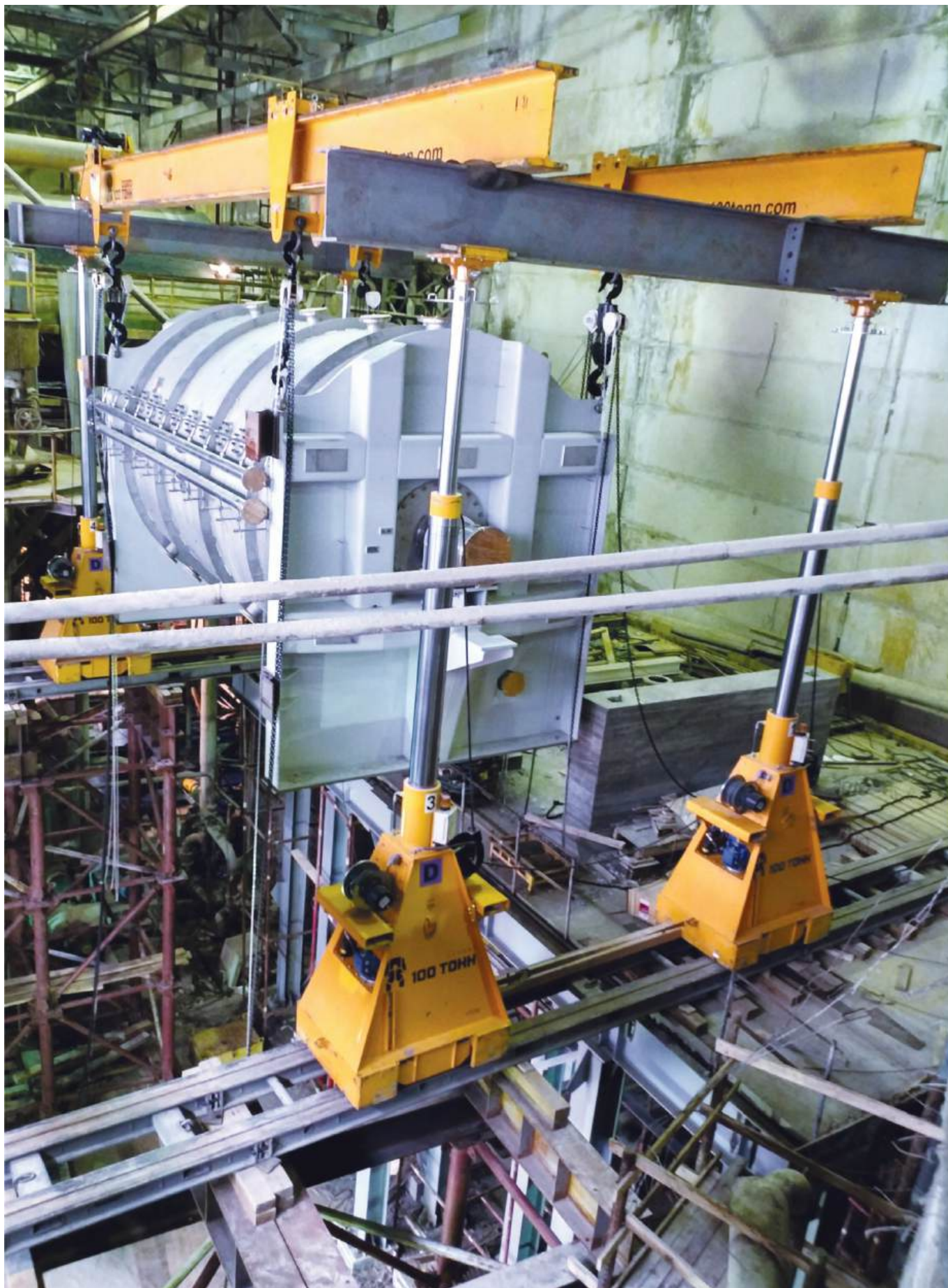
Pulp and paper mill, Novodvinsk city, Arkhangelsk region. Reconstruction of the causticization and lime regeneration plant. GP125 hydraulic gantries.
