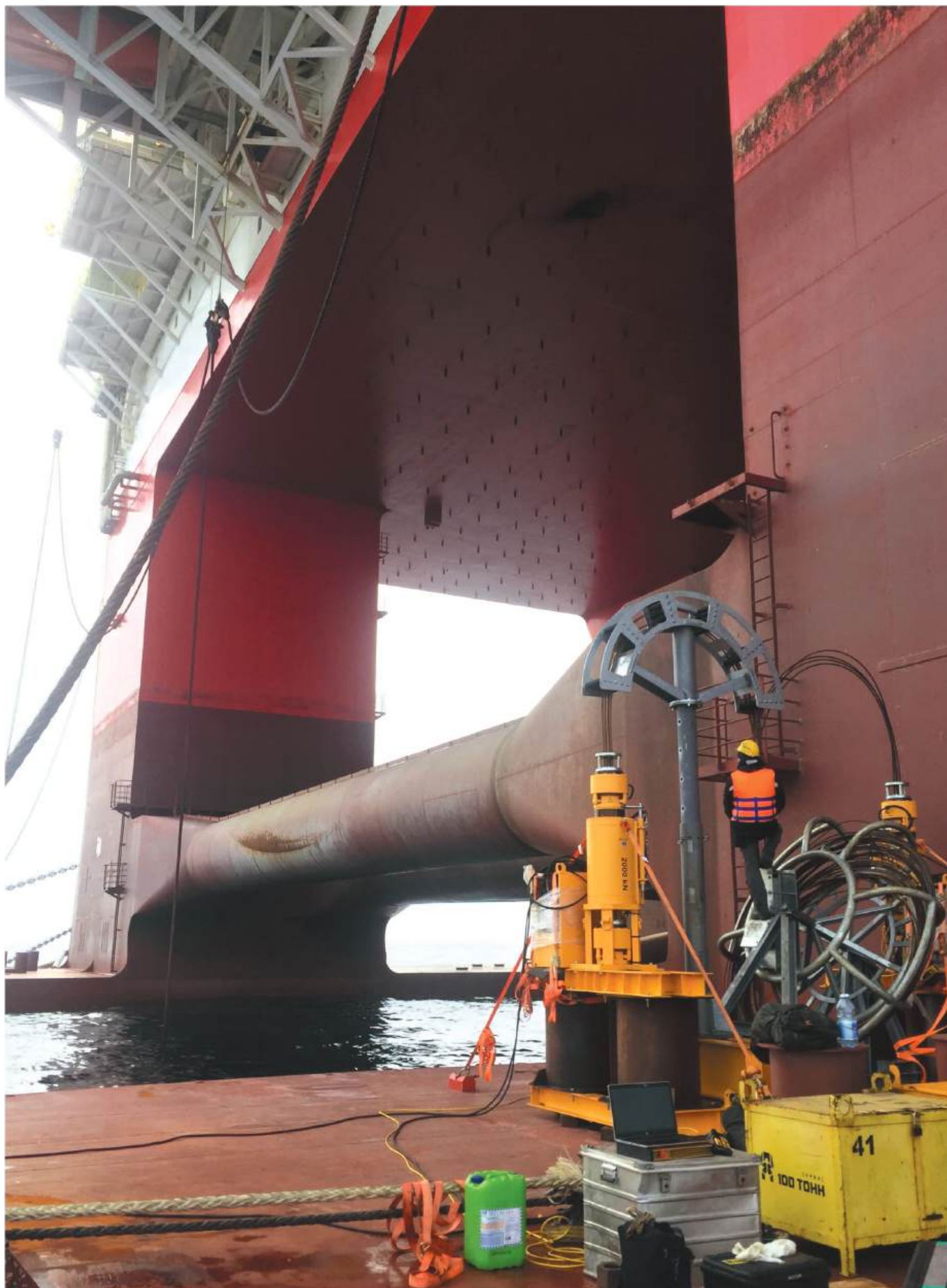
Floating drilling platform «Northern Lights», Sea of Japan. Removal of four azimuth thruster units.
