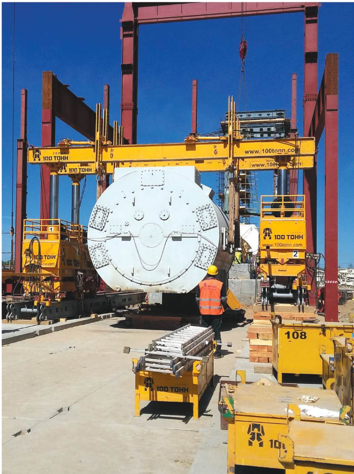
Pregolskaya Power Plant, Kaliningrad city. Installation of equipment weighing 968 tons at the same time with the construction of the turbine hall.
