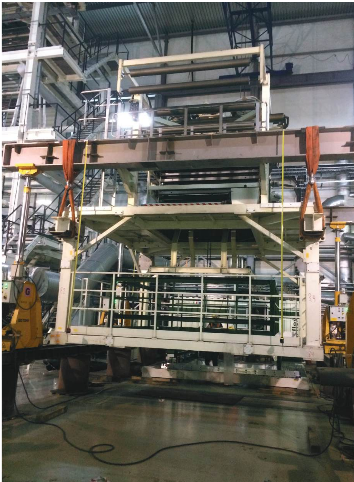
Polymer packaging manufacturing, Tashkent city. Installation and assembly of an extrusion machine. GP60 hydraulic gantries.
