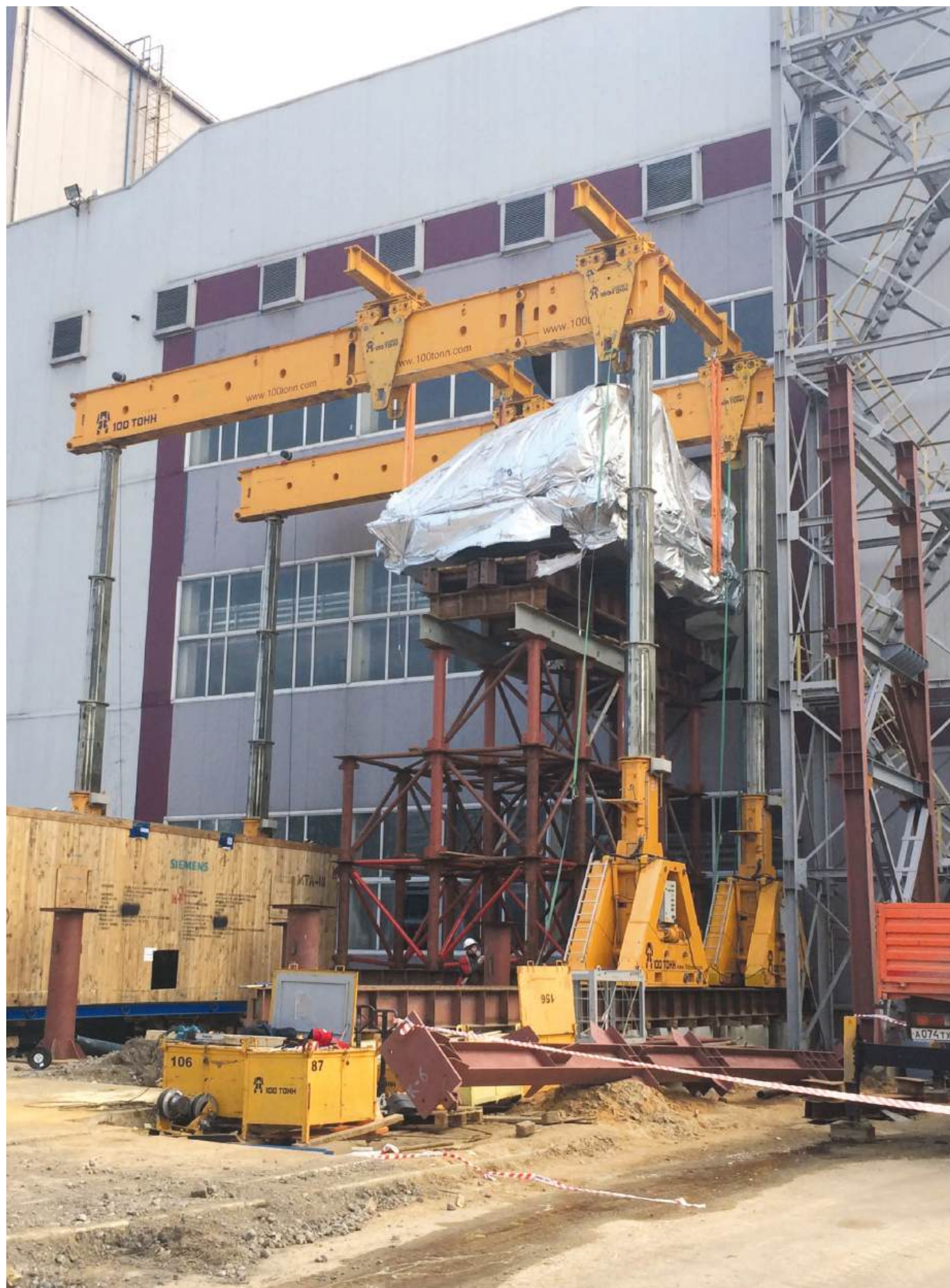
Power plant, Lipetsk city. Lifting, moving, and installing a Siemens turbine and compressor. GP1100 hydraulic gantries, modular beams.
