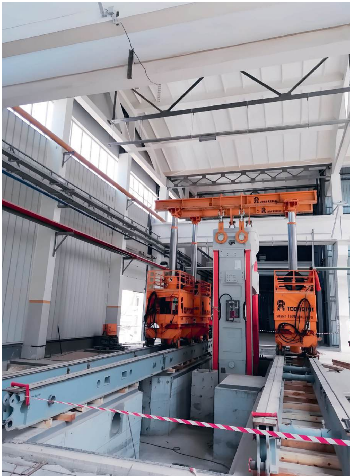
Ceramic tile factory, Samarkand city. Installation of SACMI equipment (Italy) with GP500 hydraulic gantries. Installation of two SACMI PH3200 presses, a horizontal five-deck dryer and a high-speed roller kiln.
